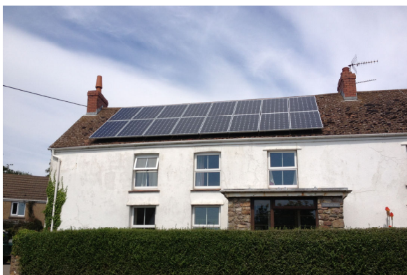
Images Top: Solar PV installation at Corn cottage, Centre: Air Source Heat Pump installation at The Laundry Bottom: Solar PV installation at Middleton Hall Farm
